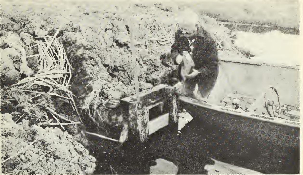
Photo 8. Redwood box type water control structure with flashboards commonly installed through interior levees for individual pond water control.
